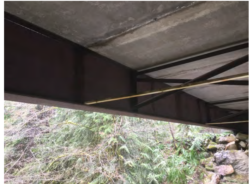
Evidence of water getting through deck joints
